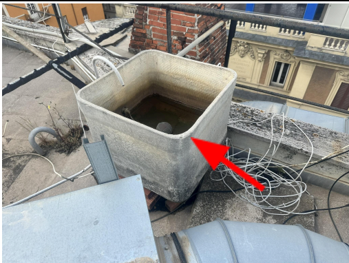
VASCA IN FIBROCEMENTO
